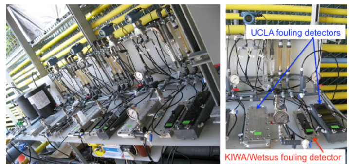
Figure 2. Research conducted at the Long Beach Water Department's seawater RO/NF demonstration plant focusing on NF/RO membrane biofouling mechanisms, prevention and monitoring. Three different membrane fouling detectors were compared to understand potential bias due to different monitoring device configurations.
